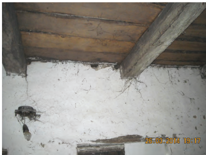
Figure 3. Nests in the cavity of a wall (original).
