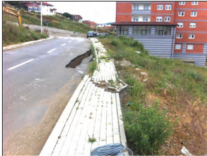
Photo 1. Landslide spot evidenced by road damages (original).
